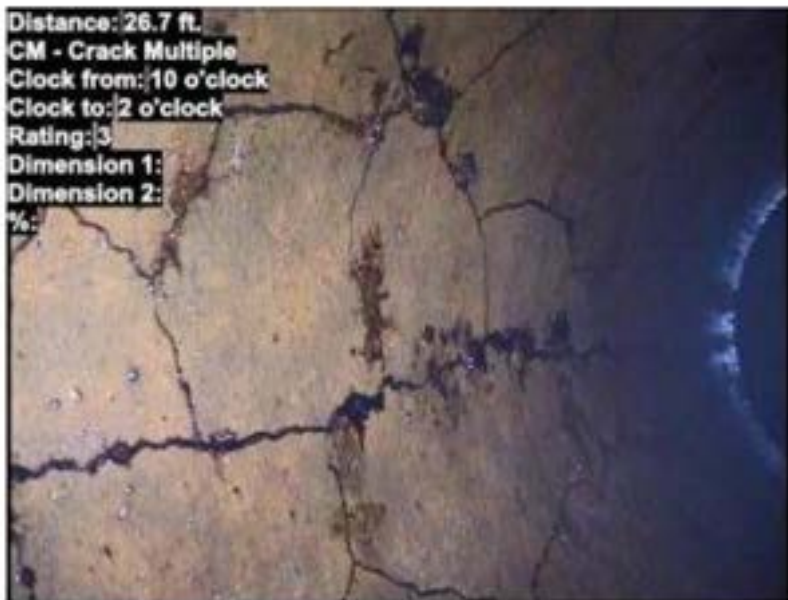
Photo Above: Cracked Sewer Pipe on Madbury Road
