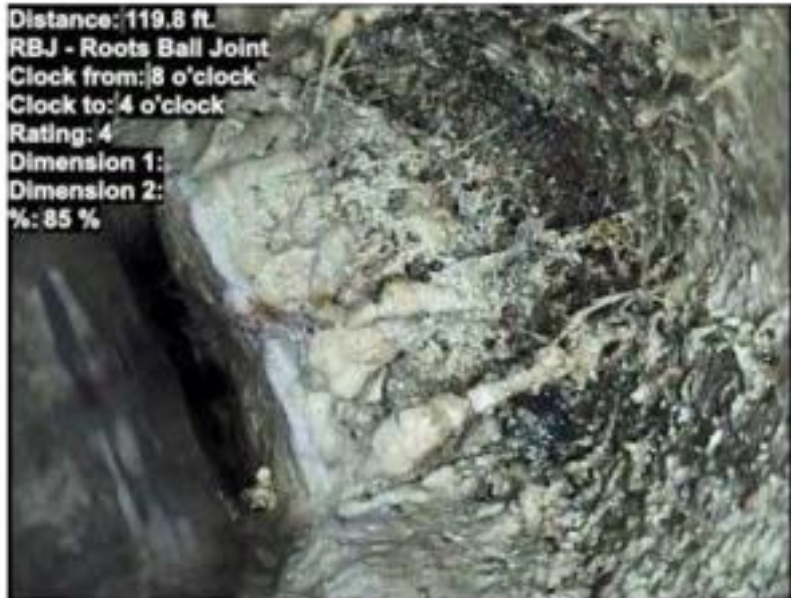
Photo Above: Root Ball at a pipe joint
